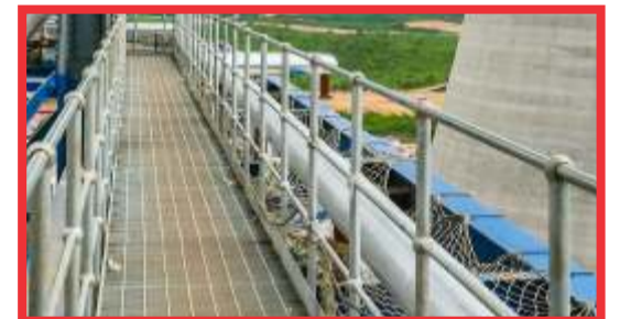
Gratings and Handrails
