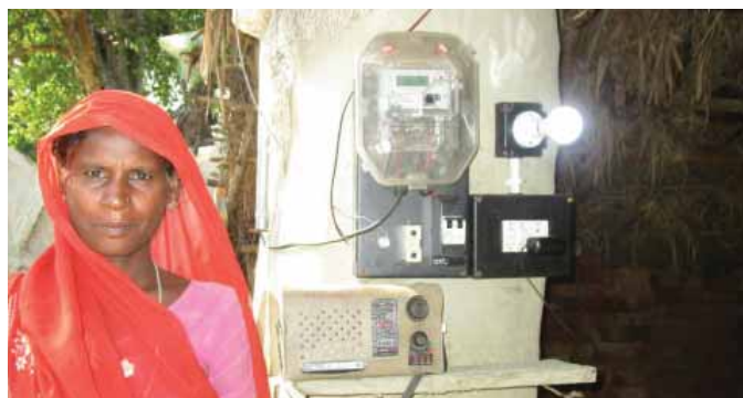
Rural household electrification under SAYBHAGYA scheme pump testing system, solar lighting system, smart meter testing, power system studies (focusing on integration of renewable energy into grid) and T&D equipment testing (e.g. transformers, cables, conductors, piercing connectors), informs Hitesh Karandikar, Director, ERDA.
