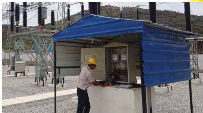
Power Quality Measurement in Power Evacuation Substation (Photo - ERDA)
